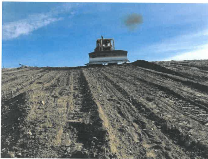
Photo B4. Spreading 12” of quality clay on track packed and compacted waste surface, Whitehorse
