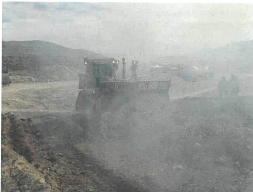
Photo 13. Clay Soil Cover Being Spread and Compacted with D7 Dozer in Tijuana Mexico Fire
