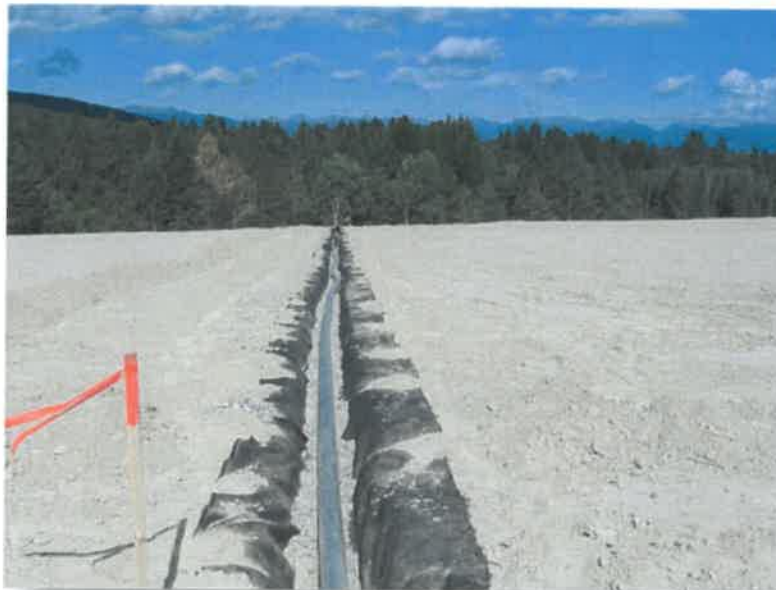
Photo 21. Typical Horizontal LFG Collector Below Cap
