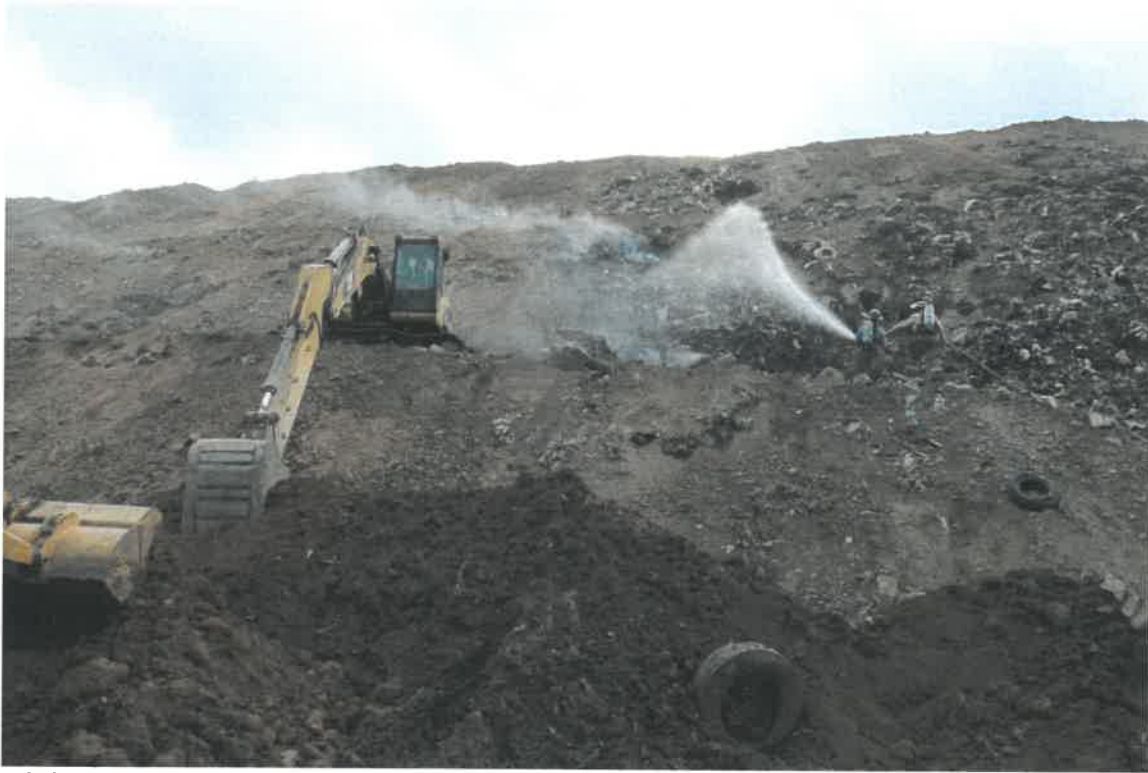
Photo B2. Very Steep Landfill Surface Being covered by dumping soil from crest. Hot spots dug out and quenched.
