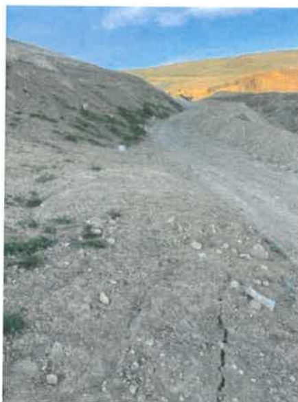
Photo 2. Slopes in Problem Area, note very steep slopes below lower bench and settlement crack
